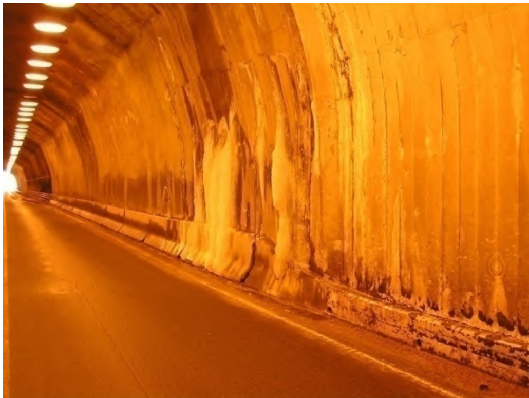
Figure 3.2 – Leakage through shotcrete liner (NCHRP, 2010).
