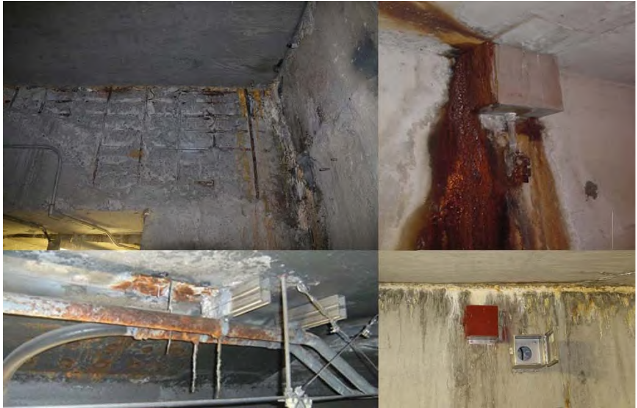
Figure 3.1 – Groundwater induced corrosion and deterioration.
