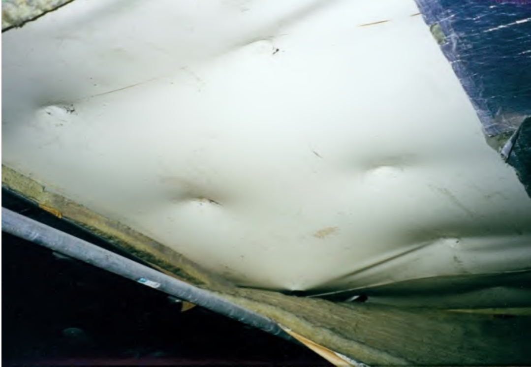
Figure 3.22 – Failed installation of waterproofing membrane in air plenum. Note that heat welded attachments did not penetrate the white waterproofing membrane (NCHRP, 2010).
