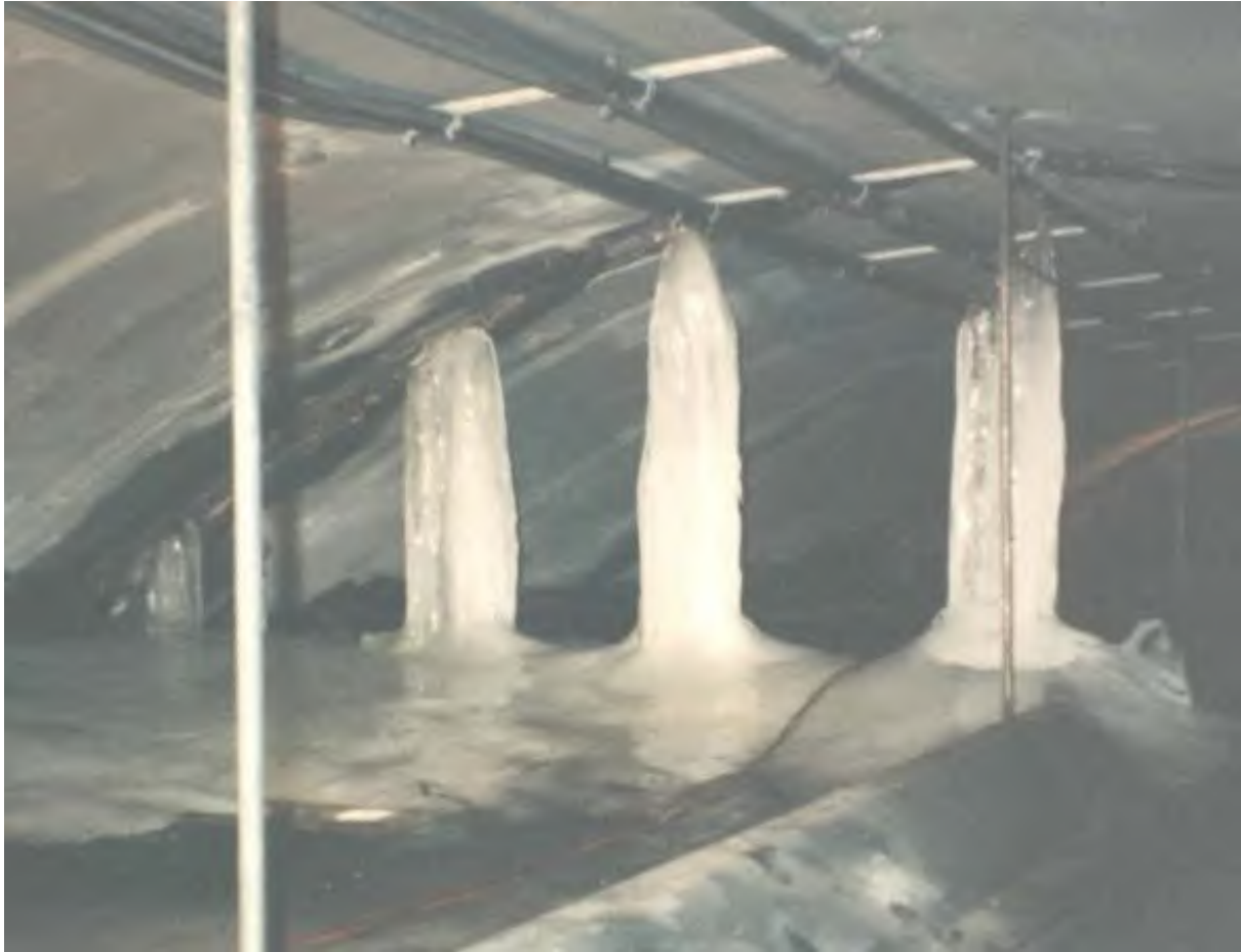
Figure 3.3 – Ice formation in plenum area above ceiling slab.
