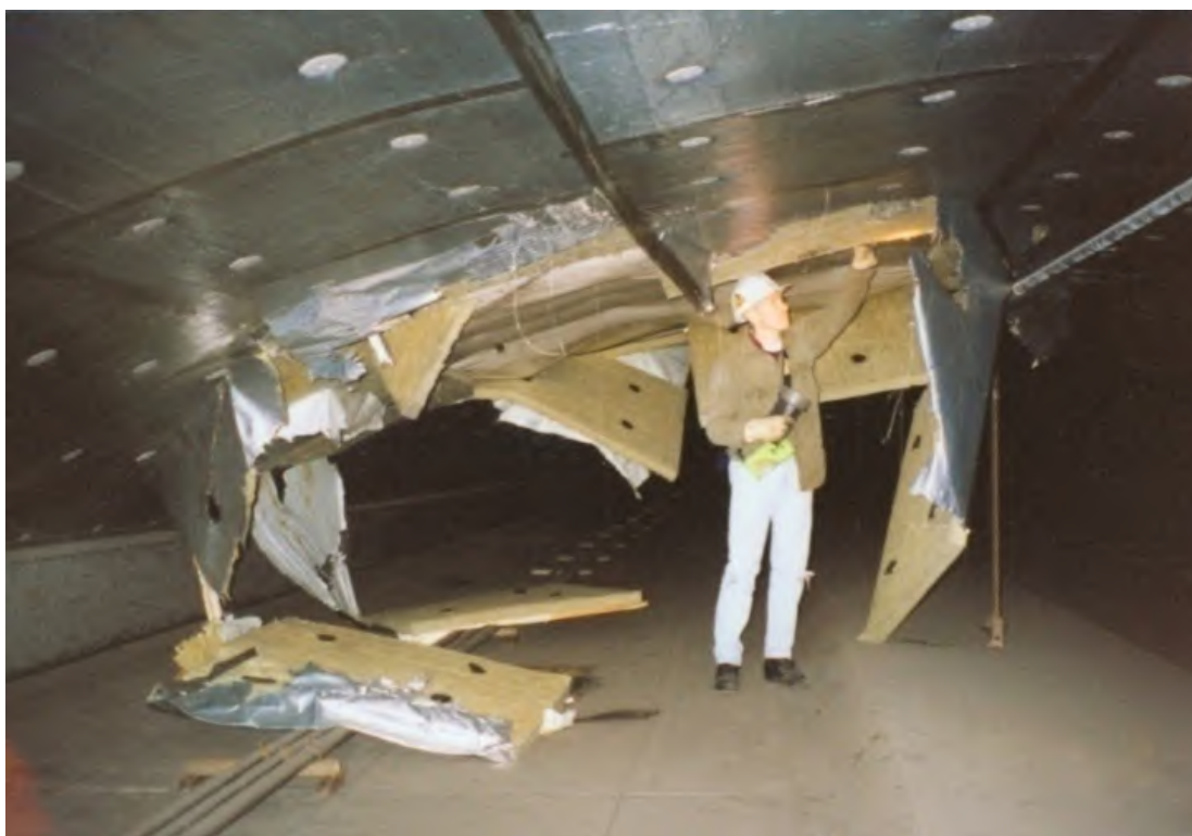
Figure 3.21 – Insulated panels under waterproofing membrane in air plenum region above roadway have dislodged in an isolated location (NCHRP, 2010).
